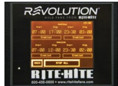
Fan network may be scheduled to start/stop twice per day
